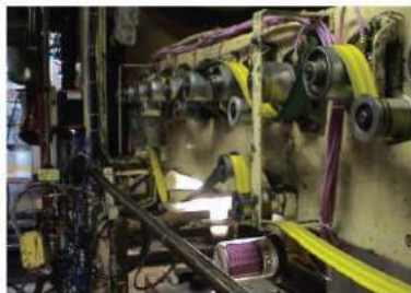
Metal industry: lubrication of return roller bearings on a production machine for aluminium sheets.
