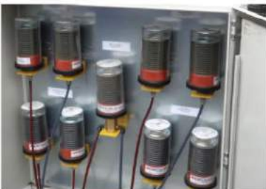
Food waste processing industry: cabinet of Memolubs for the lubrication of bearings and casing of a rotation fermenter.
